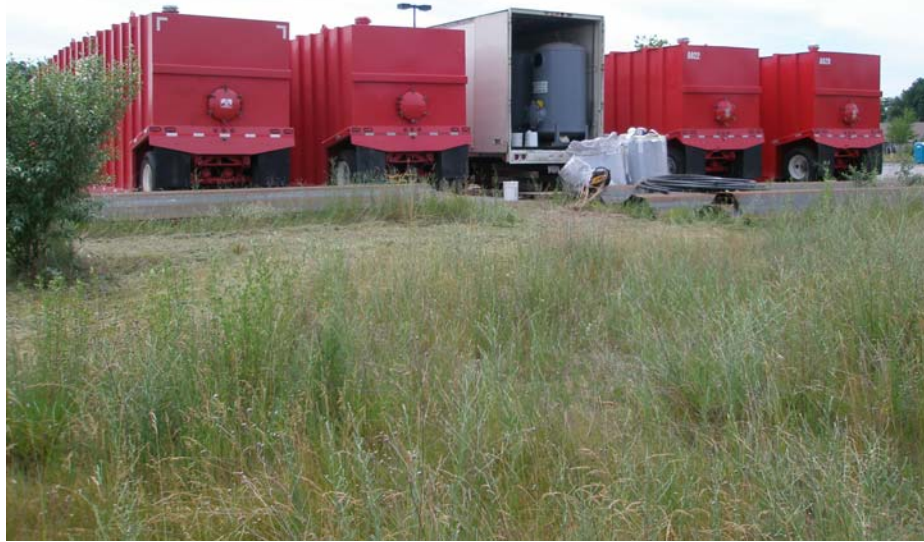
Photograph 1 – Mobile Water Treatment System
