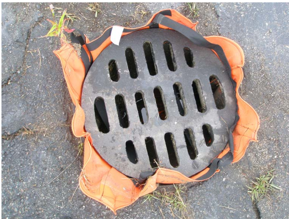
Photograph 4 – Silt Sack on Catch Basin
